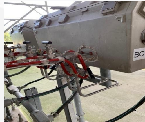
Enhanced Equipment Heat Tracing
