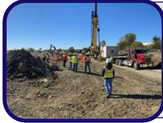
November 28, 2024 IL: Oppidan Carol Stream Data Center
